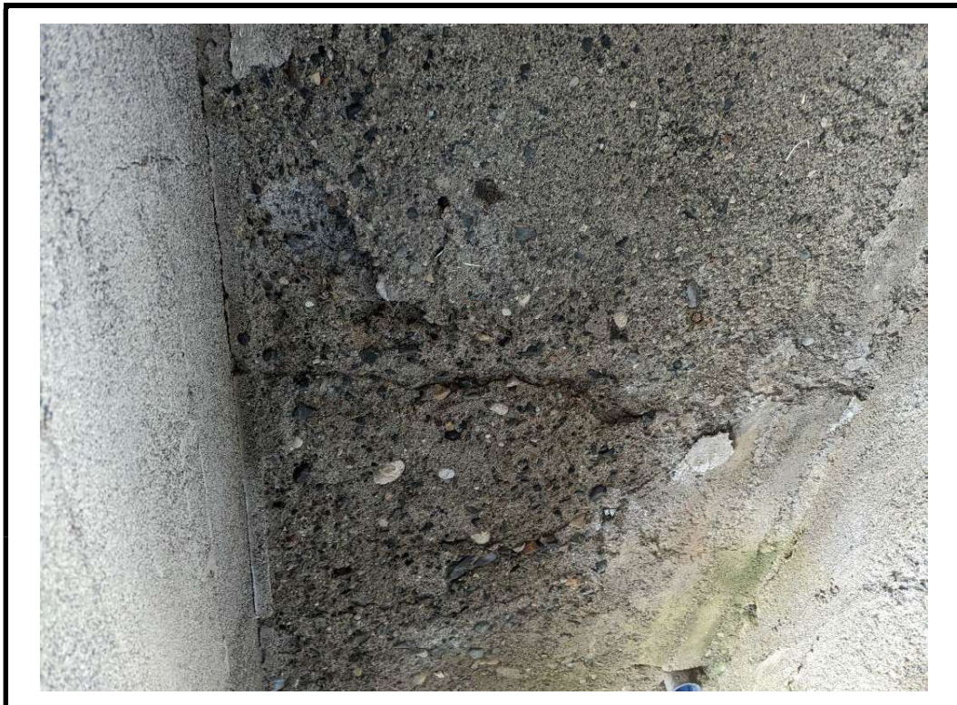
Photo 14 Moderate to severe scaling, narrow cracks and delamination noted on deck soffit
