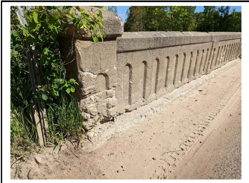
Photo 10 Moderate to severe scaling along base of north parapet wall
