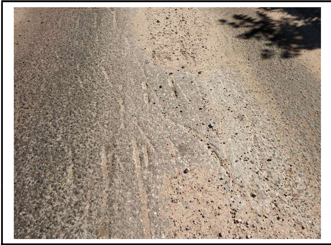
Photo 7 Moderate scaling, tire rutting and gravel accumulation in approach wearing surface (Typical)
