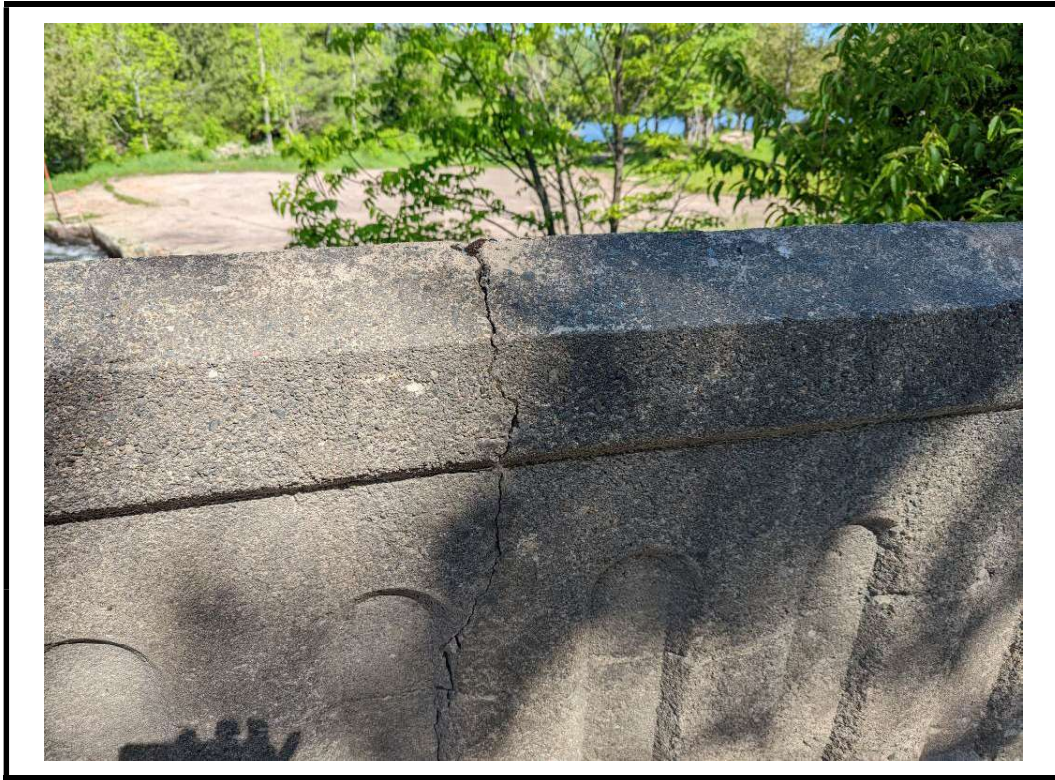
Photo 11 Medium to wide transverse crack noted on parapet wall (Typical)
