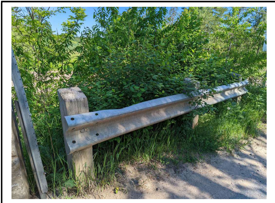
Photo 8 Typical approach barrier at northeast corner with collision damage
