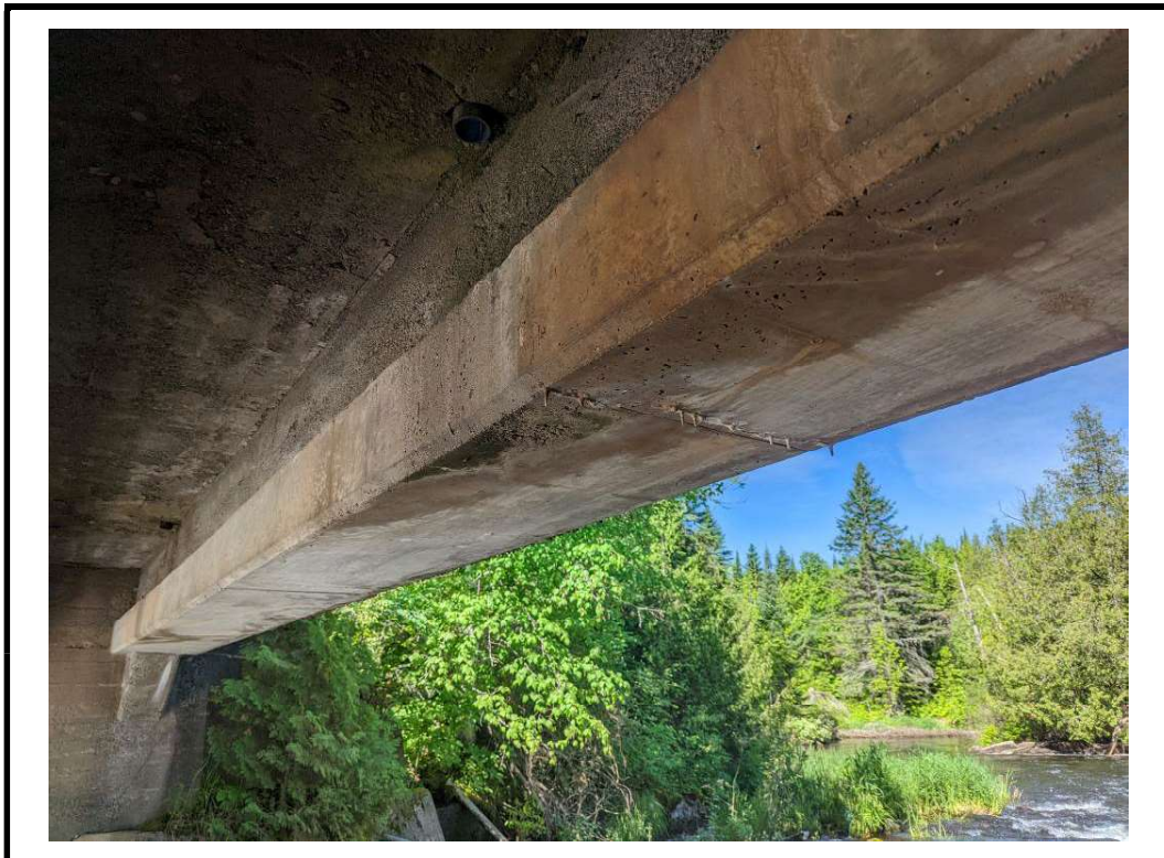
Photo 16 Stalactites observed on previous concrete repairs at girders
