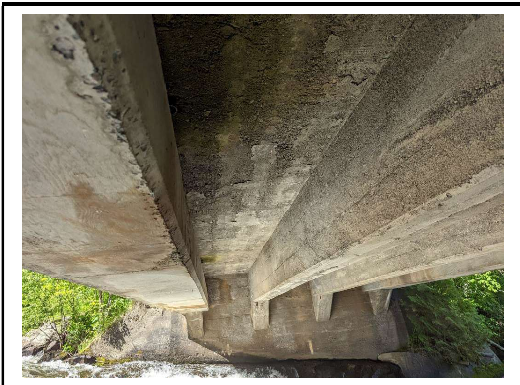
Photo 12 Light scaling on interior deck soffit
