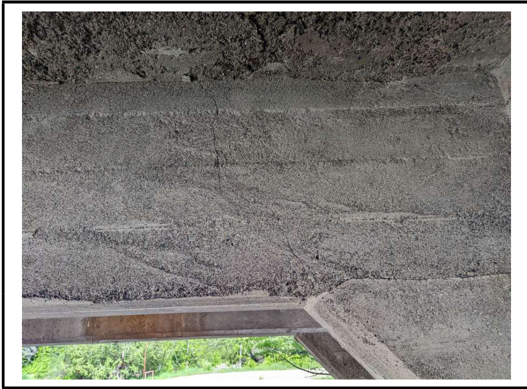
Photo 13 Narrow crack on girder
