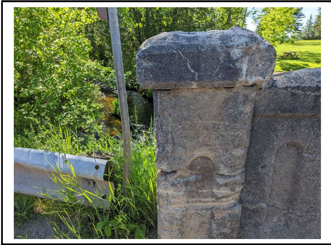
Photo 9 Substandard connection at northwest approach barrier (Typical)
