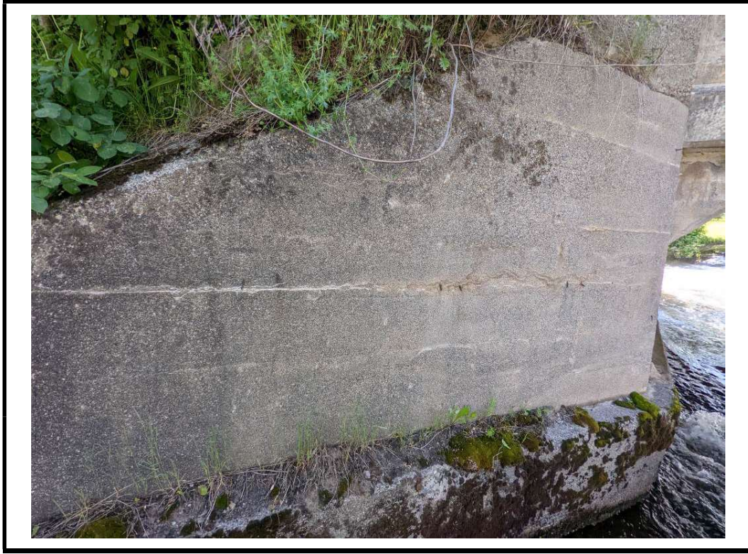
Photo 17 Narrow longitudinal and transverse cracks, damp stains and moos grown at wingwalls (Typical)
